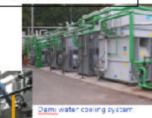
Dami water cooling system
