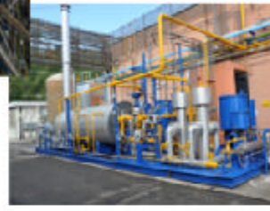
Gas heater (Forsin)
