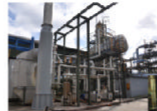
Steam generator 10 t/hr - 48 bar - 300 °C
