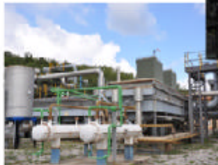
Main compressor air-aftercooler and
