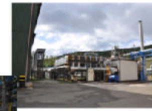
Main compressor air-intercooler
