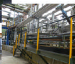
Gas pressure control valves
