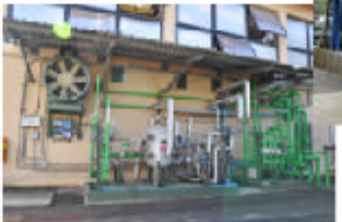
Dami water cooling system
